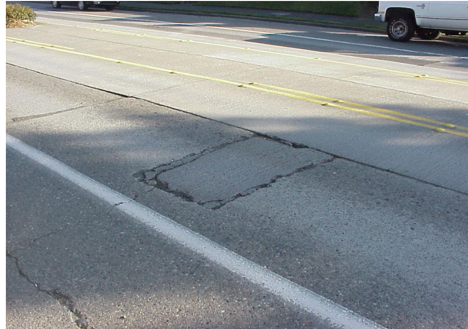
Patch with poor edges
