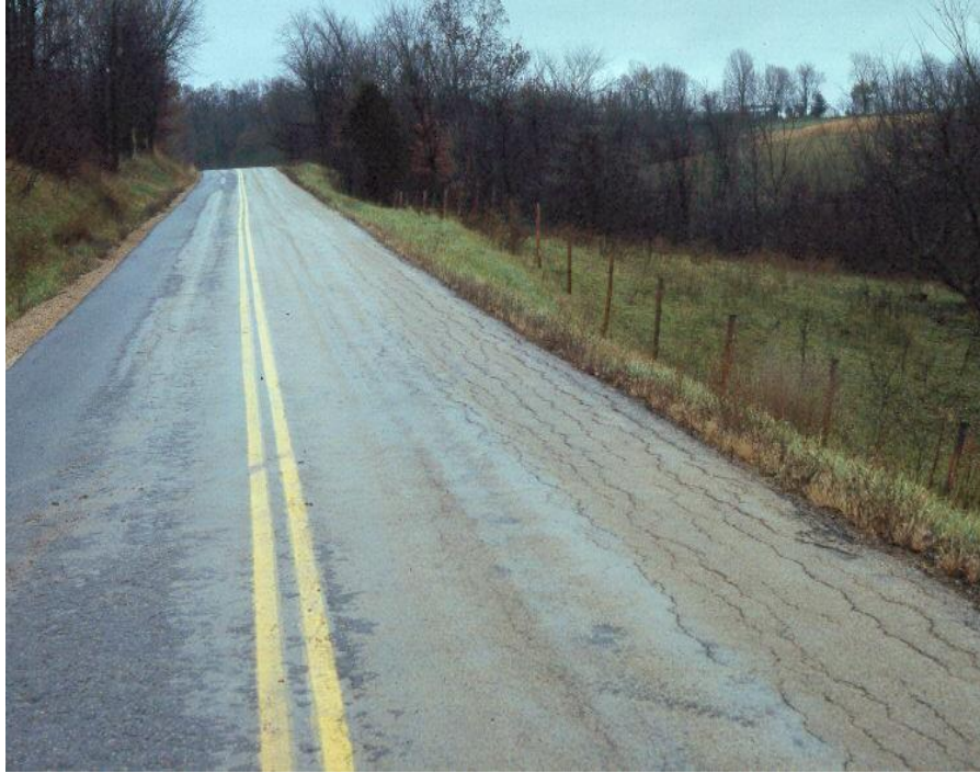
Fatigue cracking from edge failure
