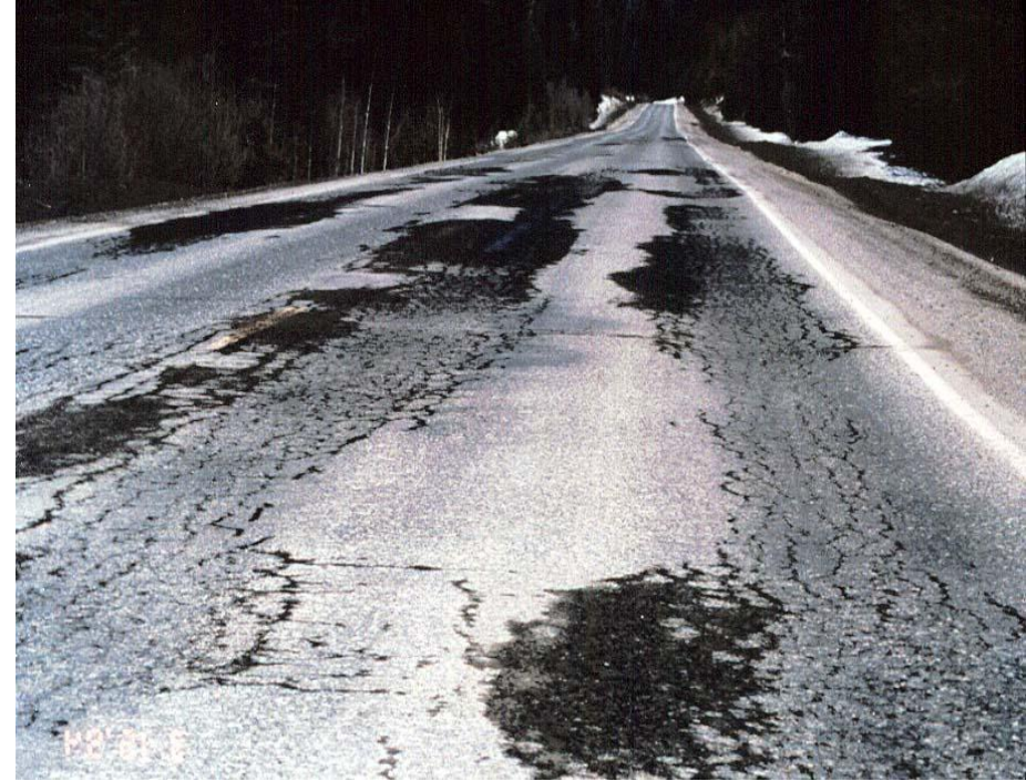
Fatigue cracking from frost action
