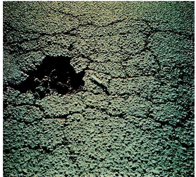
Pothole from fatigue cracking
