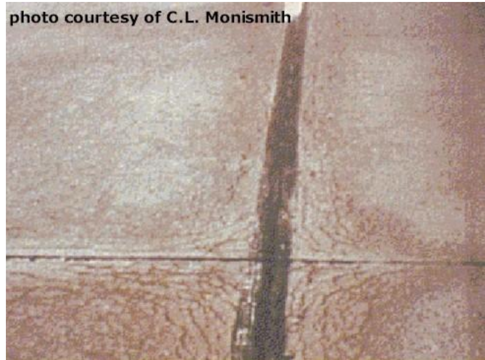
"D" cracking at panel corners
