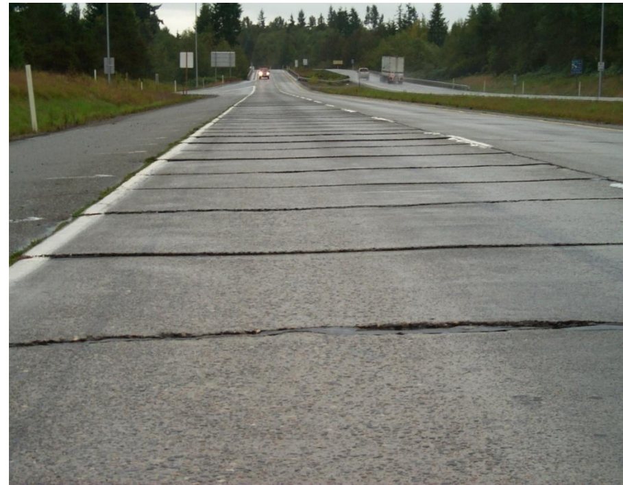
Faulting from ground level
