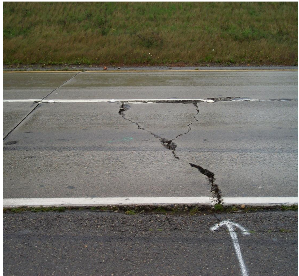
Large panel crack
