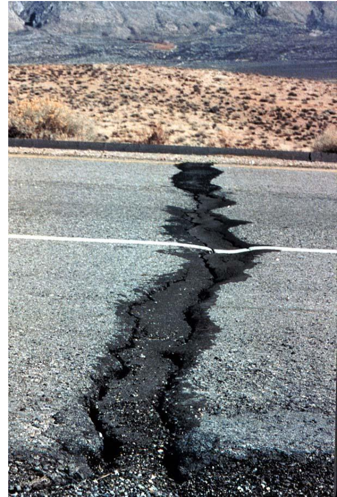
Large patched thermal crack
