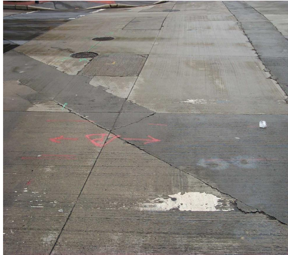
Large utility patch
