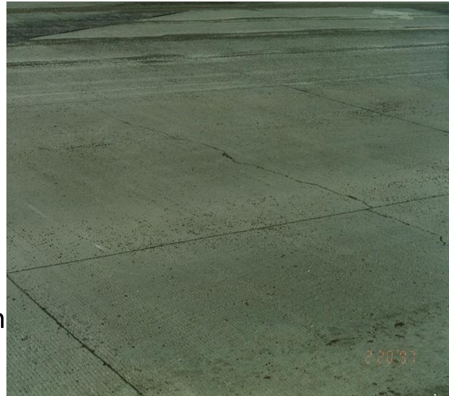
Shrinkage cracks on brand new slabs
