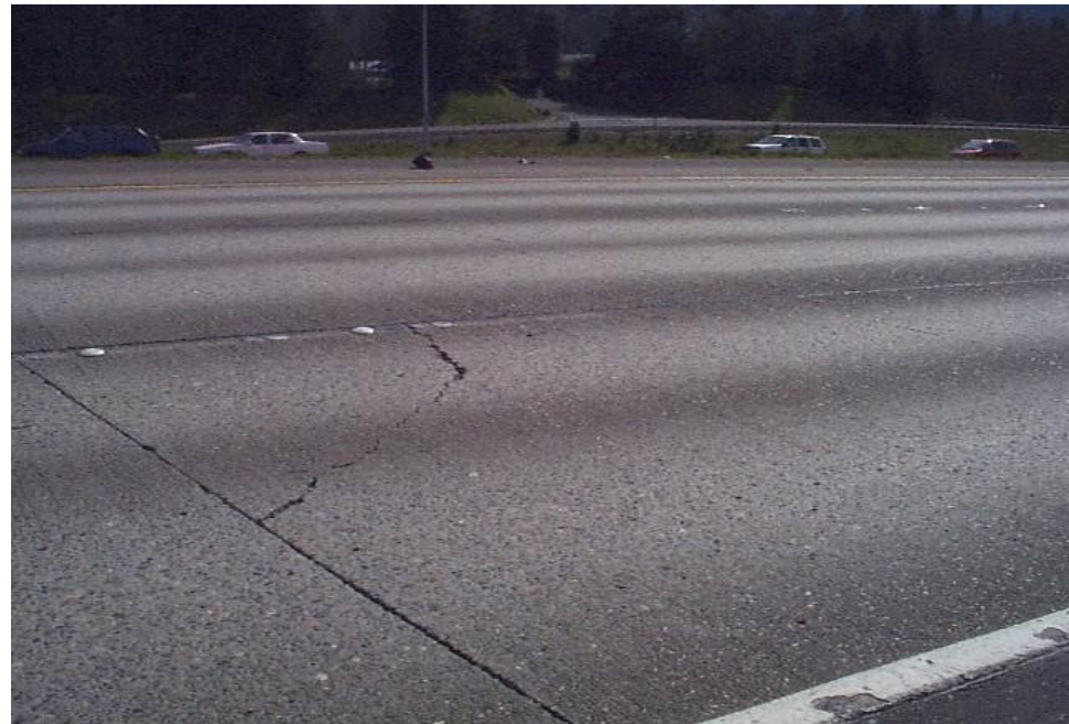
Corner break on a highway
