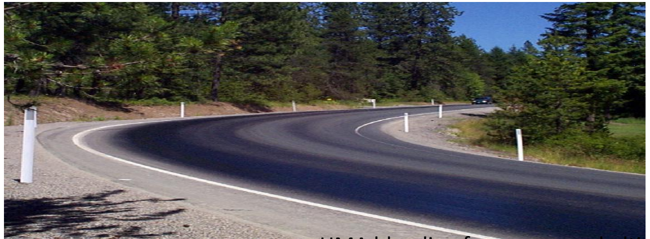
HMA bleeding from over-asphalting
