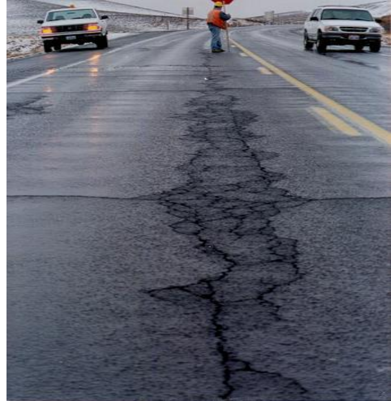
Fatigue failure from stripping
