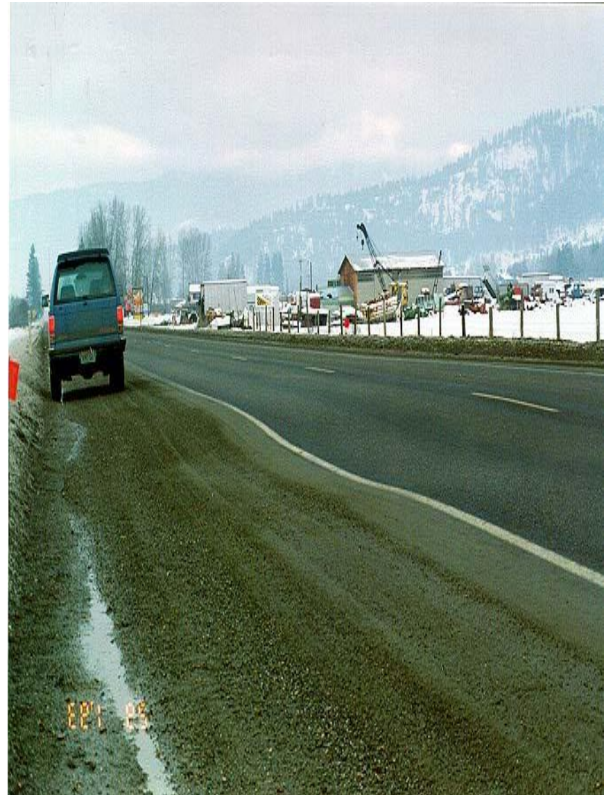
Depression in left lane and shoulder
