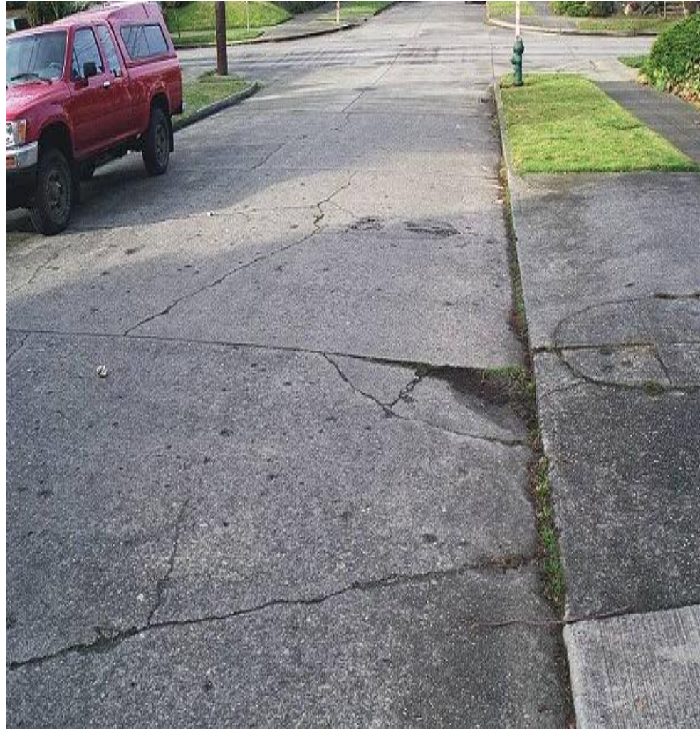
Corner break on a residential street
