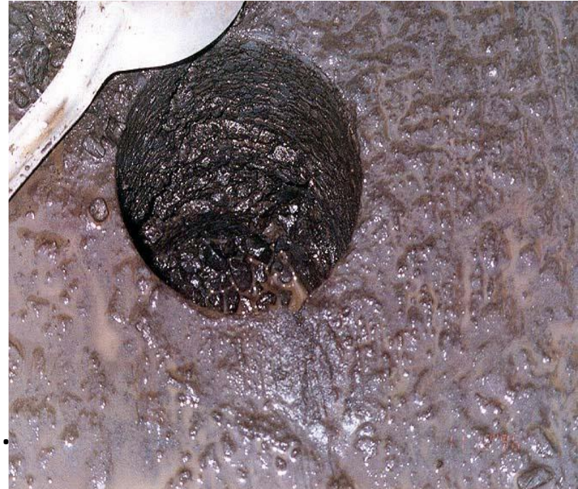
Core hole showing stripping at the bottom
