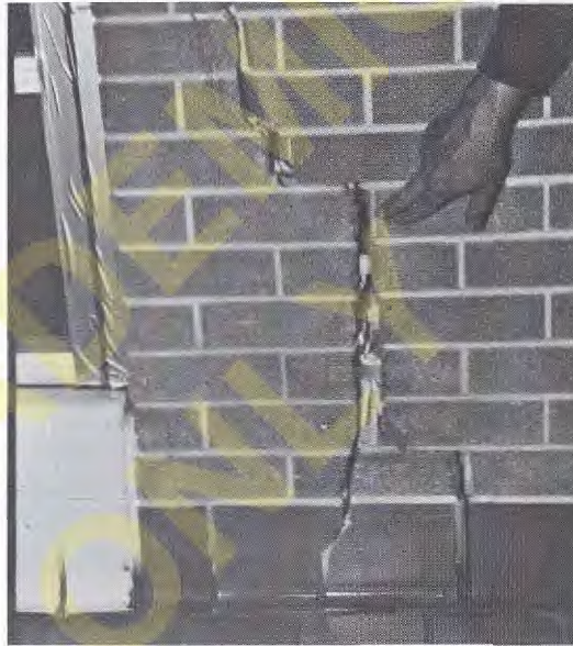
Figure 18.1 Heaving of an expansive soil caused this brick wall to crack. The $490,000 spent to repair this and other walls, ceilings, doors, and windows represented nearly one-third of the original cost of the six-year-old building (Colorado Geological Survey).
