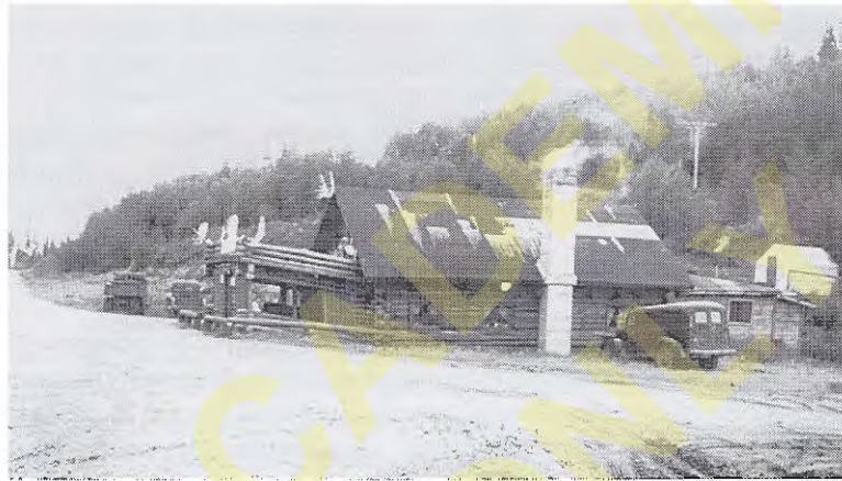
Figure 18.6 Heat from this lodge in Alaska thawed the permafrost below, causing it to settle. However, the permafrost did not thaw beneath the unheated porch (Photo courtesy of Professor Richard L. Handy).
