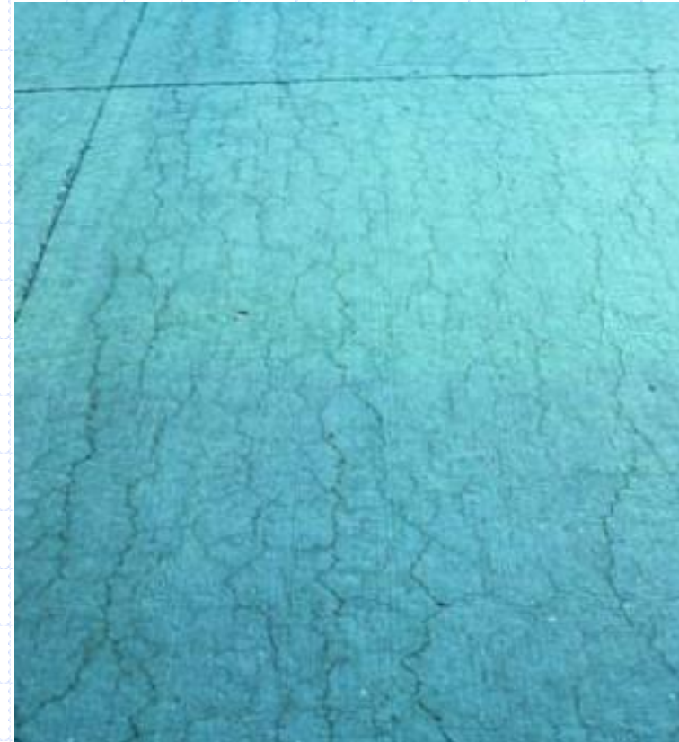
AAR Induced Cracking in Concrete Pavement.
