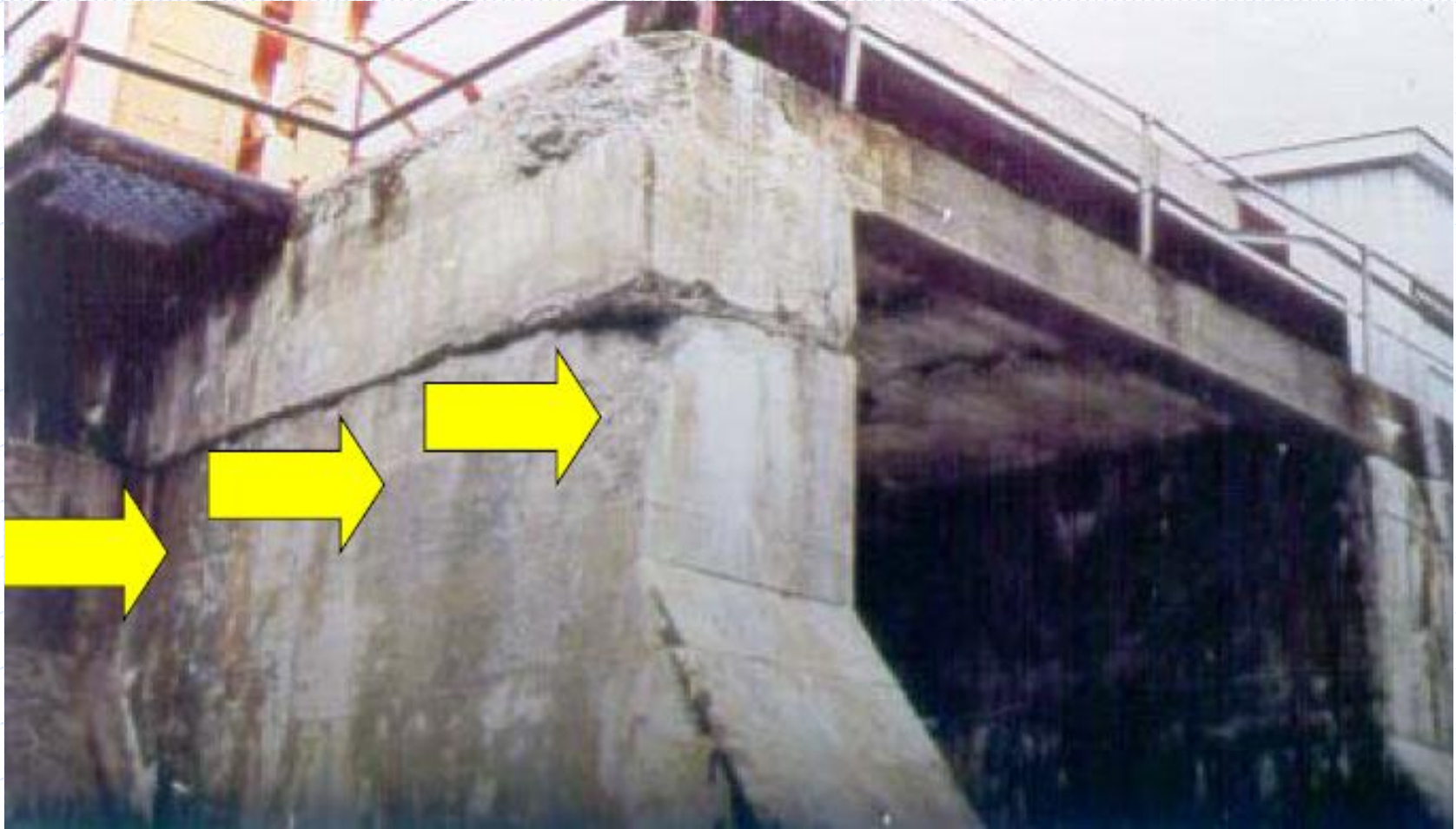
Displacement caused by AAR induced expansion in Dam structure
