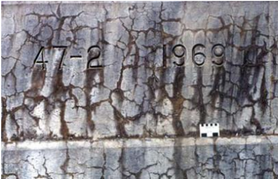
Map cracking and discoloration due to ASR – Parapet wall, Northern Ontario
