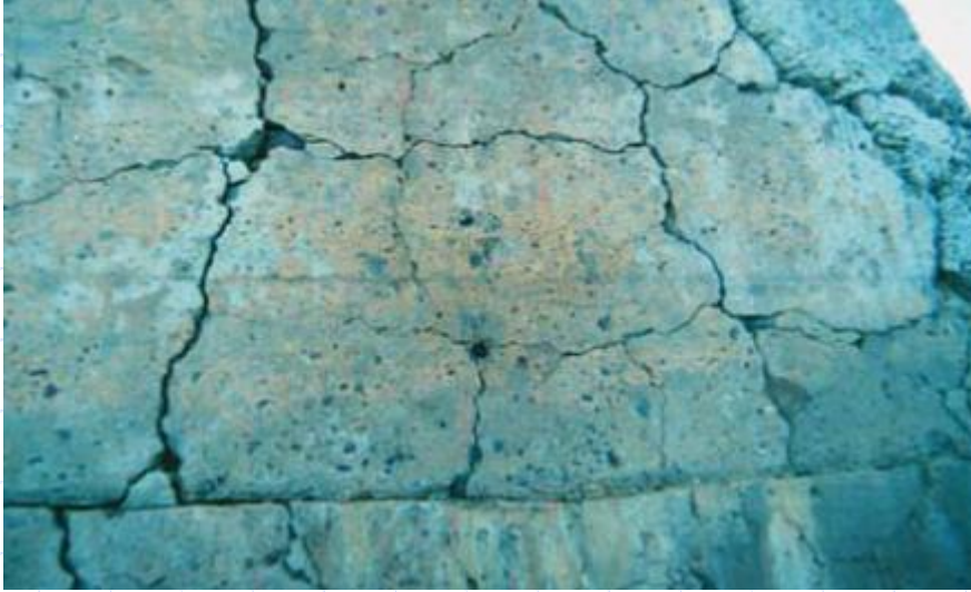
Map cracking pattern Bridge Pier, Medicine Hat, Alberta
