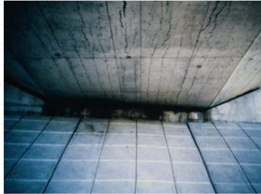
ASR Induced Longitudinal Cracking in Soffit of Bridge Deck
