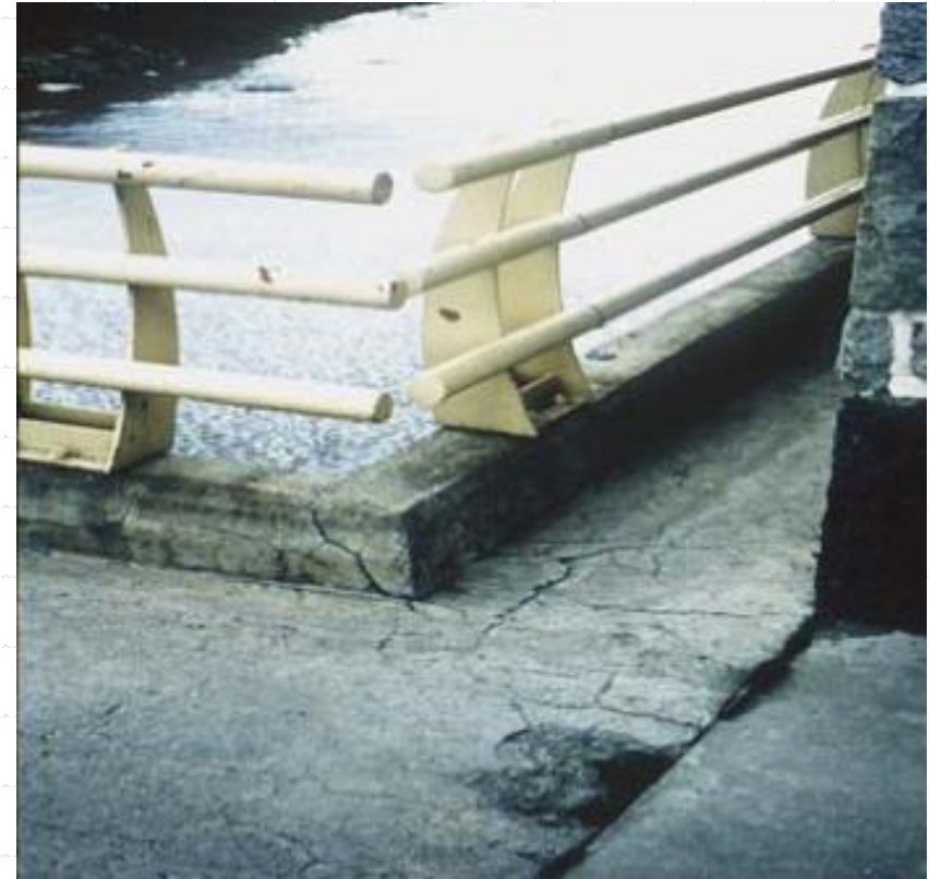
Displacement caused by ASR-induced expansion in bridge structure; spalling and extrusion of jointing material
