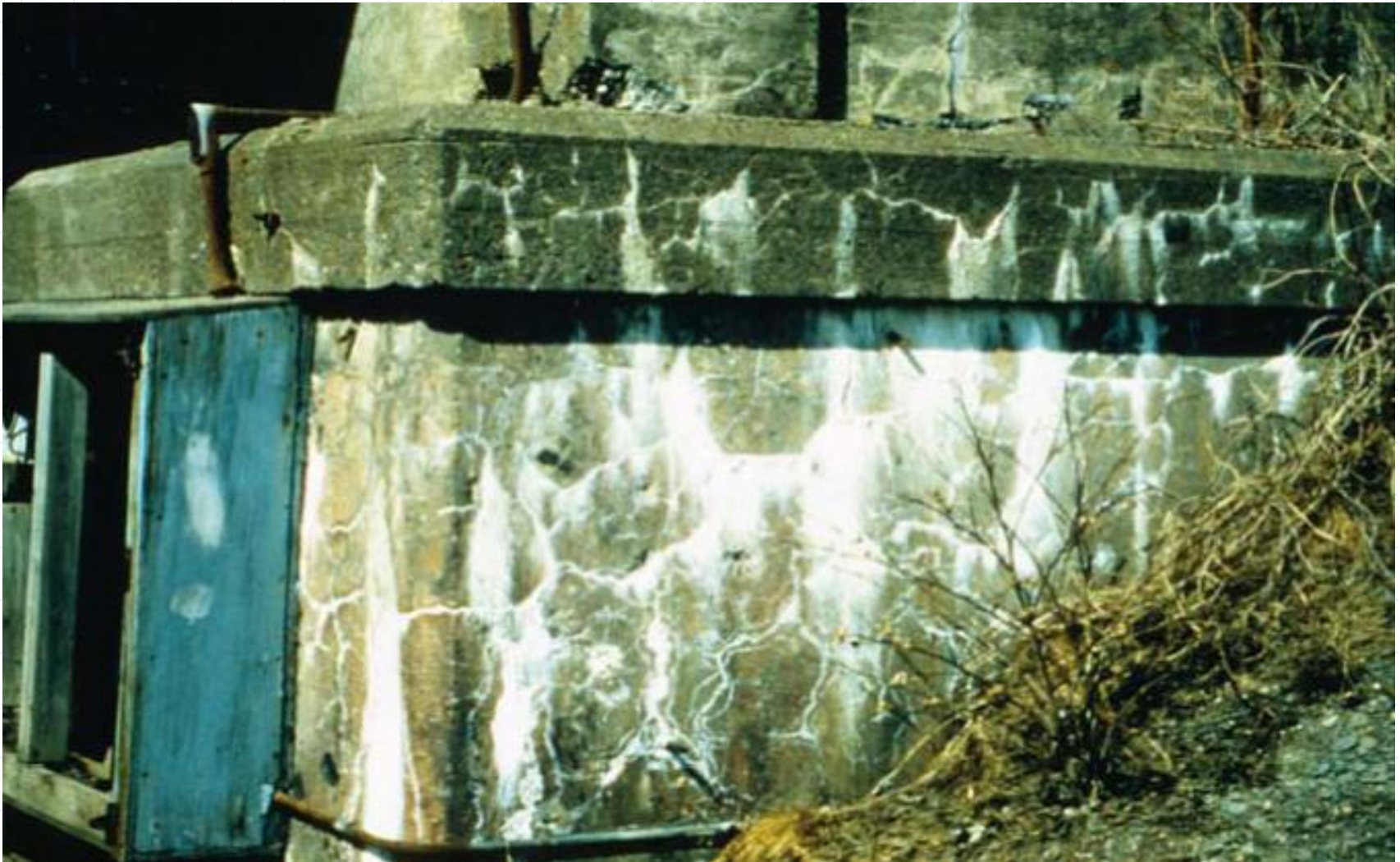
Exudations of alkali-silica gel - Bridge Foundation, Nova Scotia
