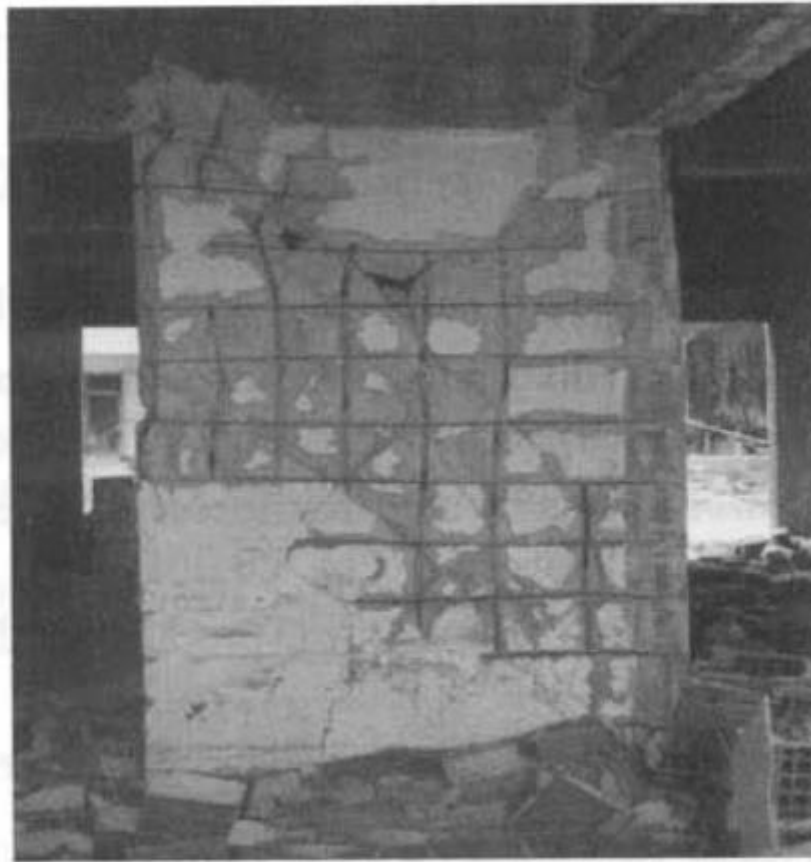
Shear wall after an earthquake.
