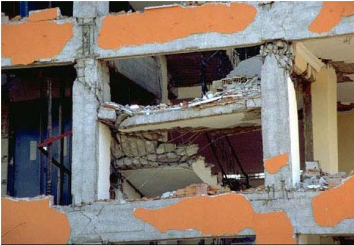
Figure 3-48 Damage at the rear stairwell
