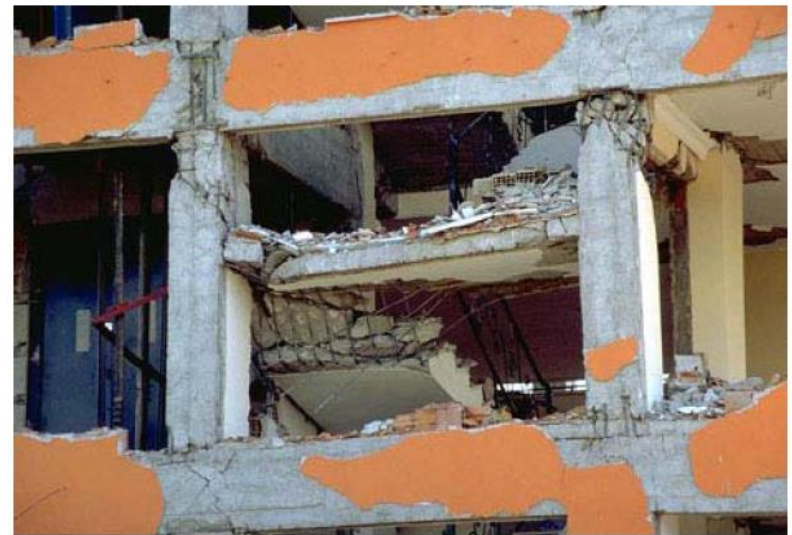
Figure 3-48 Damage at the rear stairwell
