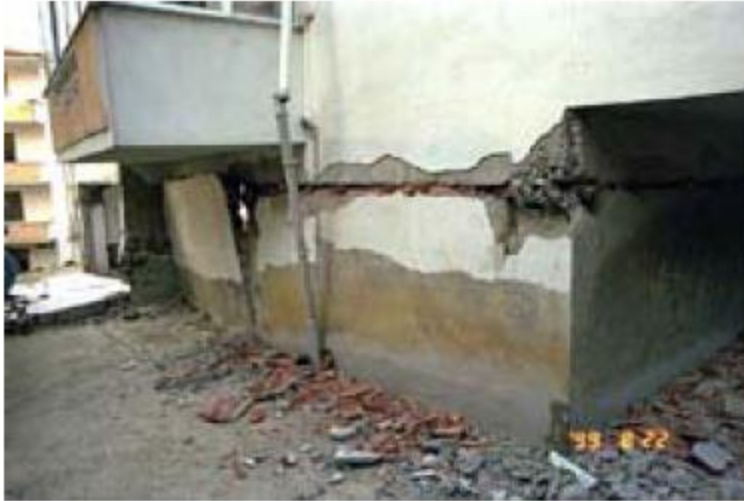
a. damage from out-of-plane deformation
