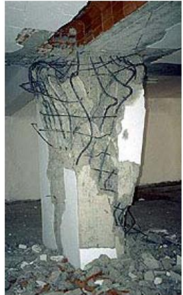
Figure 3-50 Axial failure of column B (See Figure 3-46)
