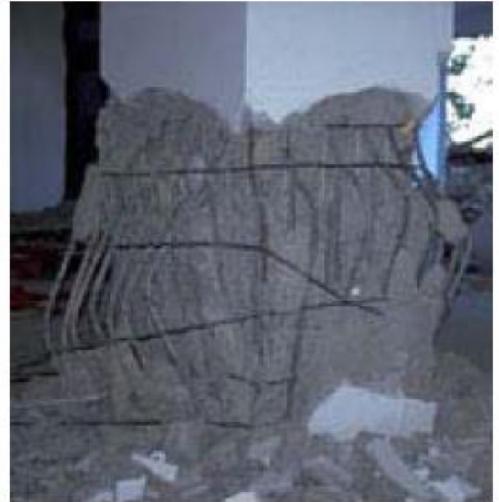
Figure 3-51 Axial failure at lap splice in Column C (See Figure 3-46)
