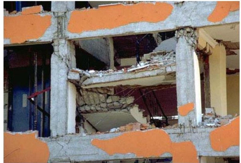
Figure 3-48 Damage at the rear stairwell
