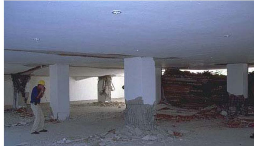
Figure 3-47 Damage to first story columns
