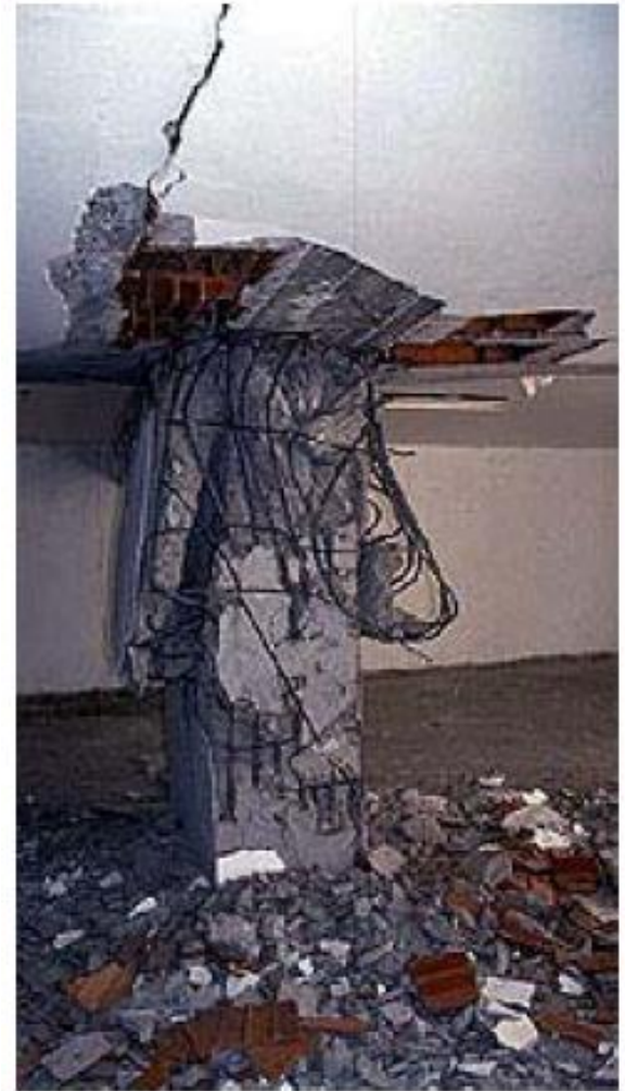
Figure 3-49 Shear failure of Column A (See Figure 3-46)
