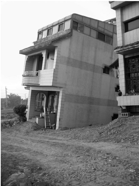
Figure 3-12. Liquefaction-induced tilting of three-story residential structure in Central Taiwan. Photograph by Dr. Farzad Naeim.
